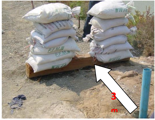
Figure 3.5 To set the wooden plank and sand bag 3.0 meters from a borehole
